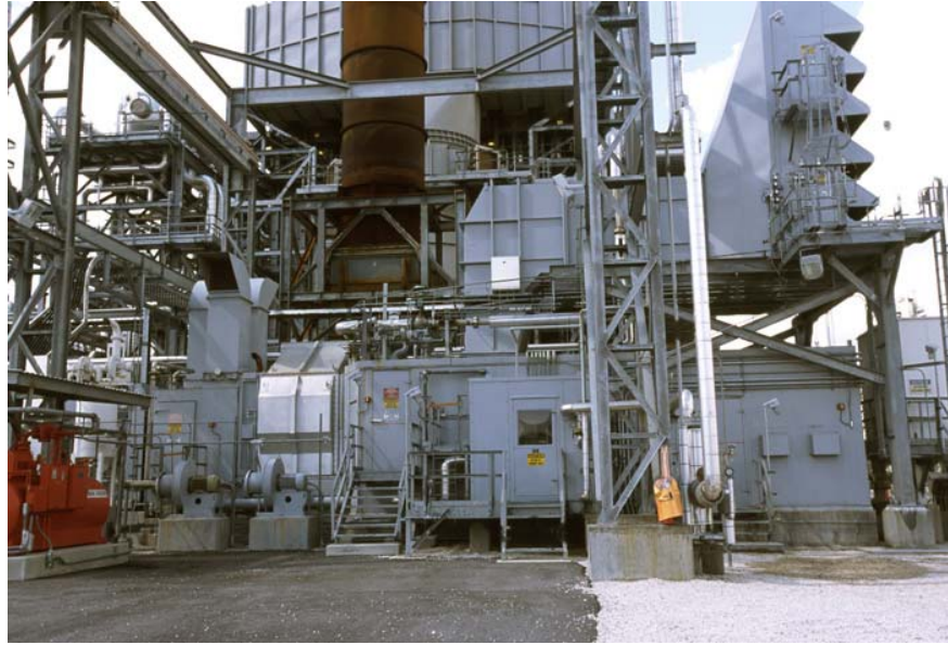
Figure 2: Photograph of Gas Turbine at the Air Products Port Arthur Plant
