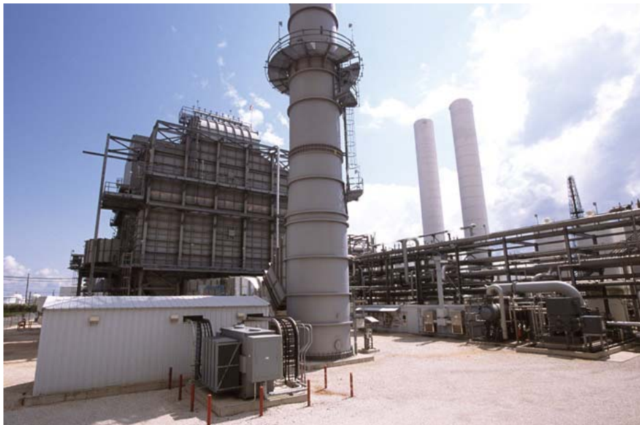
Figure 1: Photograph of the Air Products Port Arthur Hydrogen Plant
